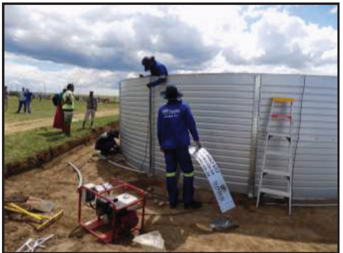
A 112kl tank was erected in order to relieve the devastating need for water in Ntha.
