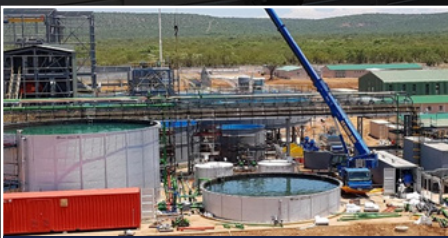
Process Water Storage
