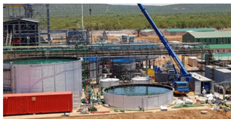
Mine infrastructure integration
